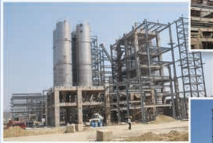
Polypropylene Unit with four Pellet Blending Silos
