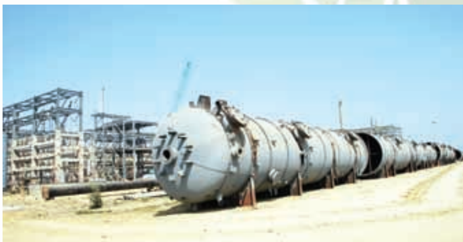
Arrival of Propylene Fractionator No. 2 sections, the tallest equipment in the plant
