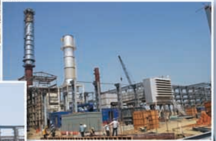
The Captive Power Plant
