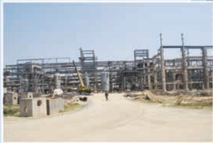
The Ethylene Cracker Unit
